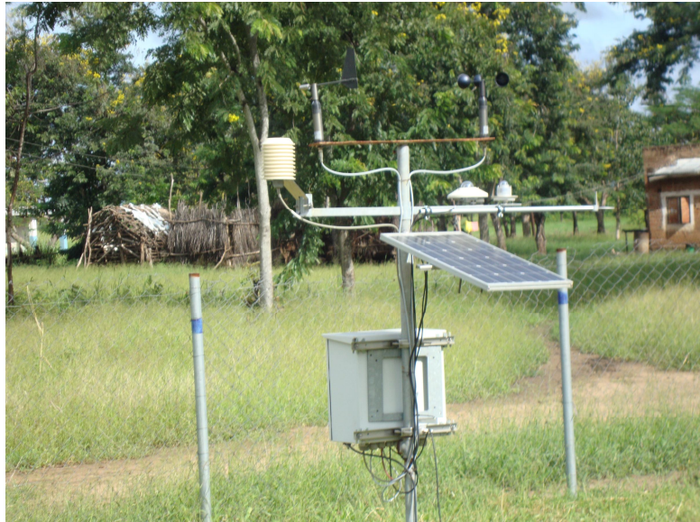
Figure 4.9 Mkindo Automatic Meteorological Station
