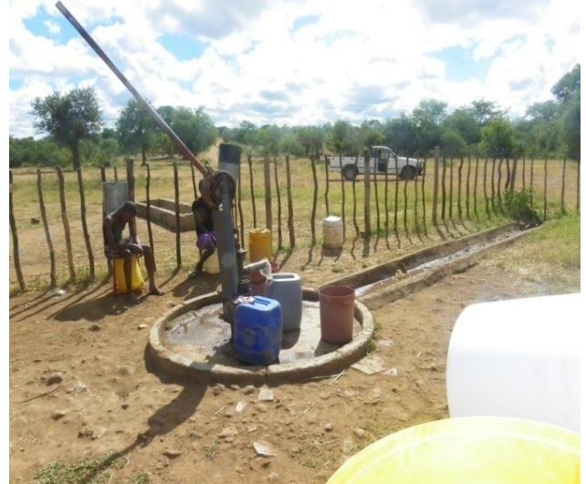
(b) Mpasikwe Borehole in Ward 2 fitted with type C bush pump
