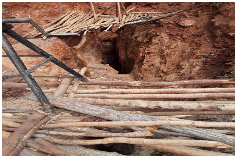
Plate 6: The use of timber in primary construction of mining shafts. Source: M. Jomboro, 2018.
