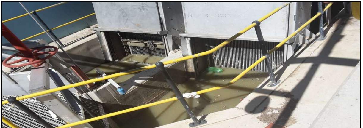
Figure 2-3: Screen at Gammams wastewater treatment plant
